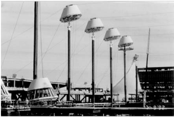
Steel masts were guyed with external temporary cables, and truss rings were assembled around mast bases and winched up into position.
