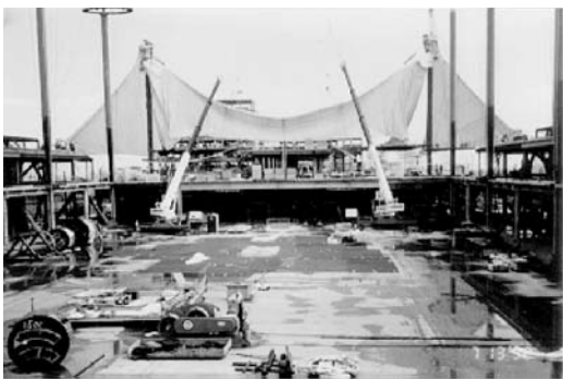
Fabric was lifted into place with a drum hoist (in foreground) secured on the terminal's Main Level 5. Two hydraulic cranes were also used to assist with the lifts.
